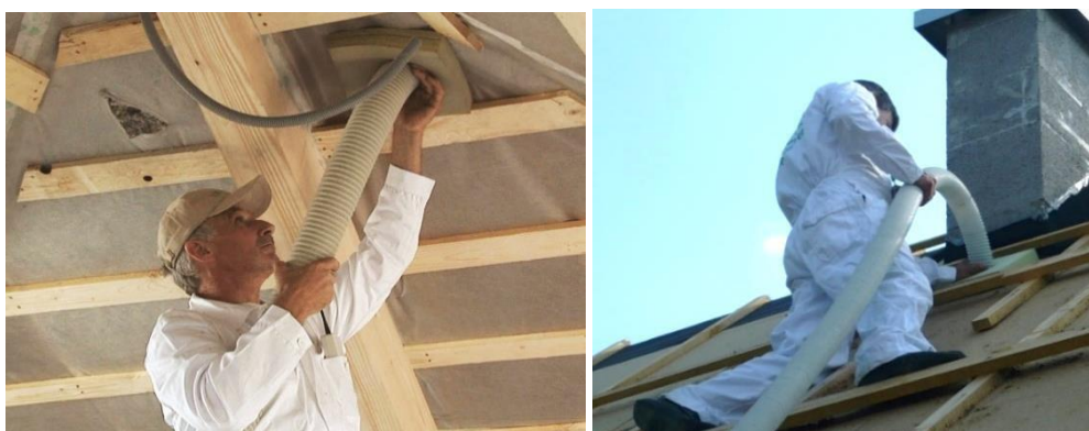
Figure 3: Cellulose insulation in a pitched roof
